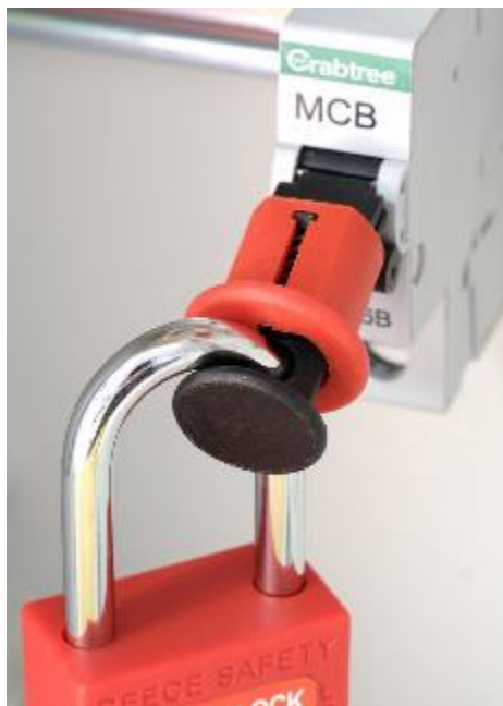
Lock-out devices in use
